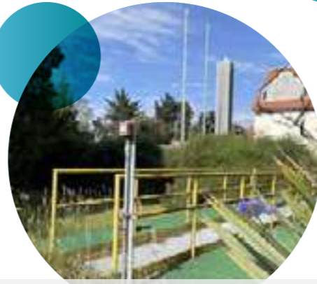
Gas Compression Station La Sabana
